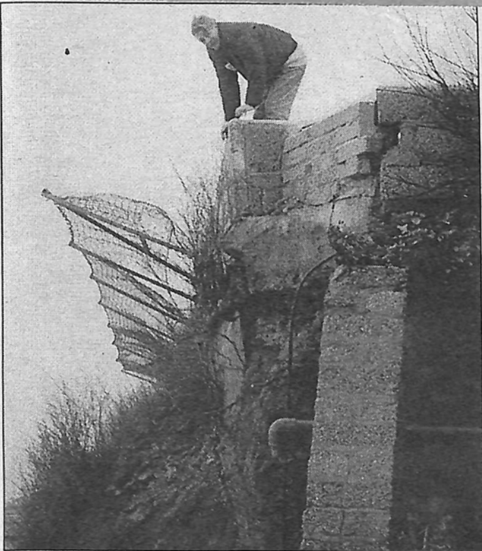
Richard Palmer of the Tye Rock Hotel, Porthleven, stands at the edge of the swimming pool which is in danger of collapsing as the cliff underneath it has subsided
