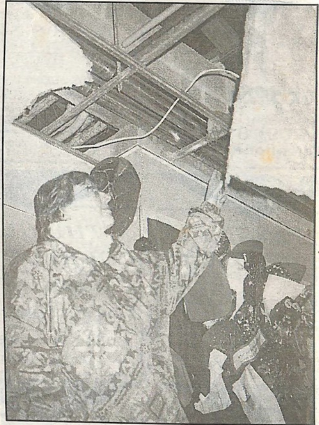
□ Headteacher at Porthleven, Helen Williams, inspects a damaged ceiling in a classroom.
